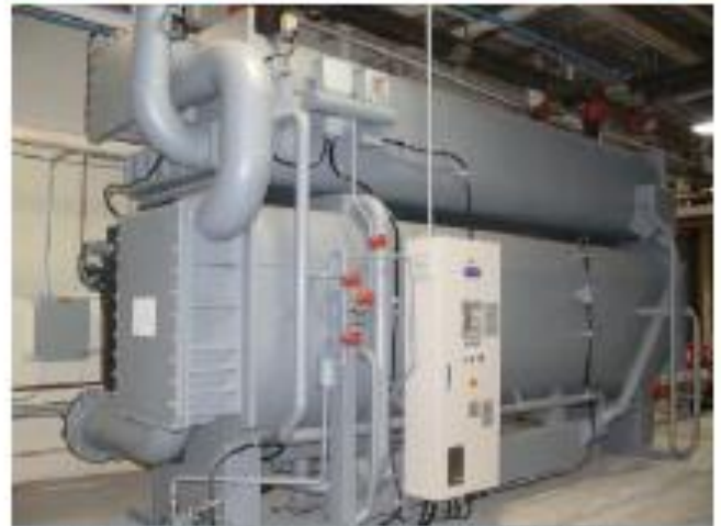
A 400-ton single-stage absorption chiller integrated with three 600 kW reciprocating engines provides hot water for process and space heating. The system is located at a metal fabrication facility in Fitchburg, Massachusetts. Photo courtesy of Northeast CHP Technical Assistance Partnership (CHP TAP).
